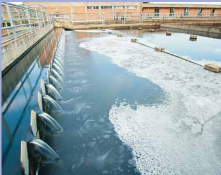
Bathurst filtration plant
